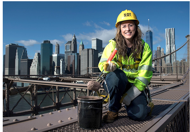
Elisangela “Lisa” Oliveira is a bridge painter for the New York City Department of Transportation.
